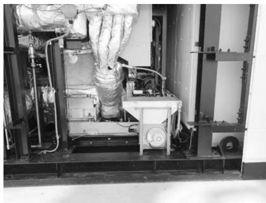
Fig. 13 MGT installed in SOFC
